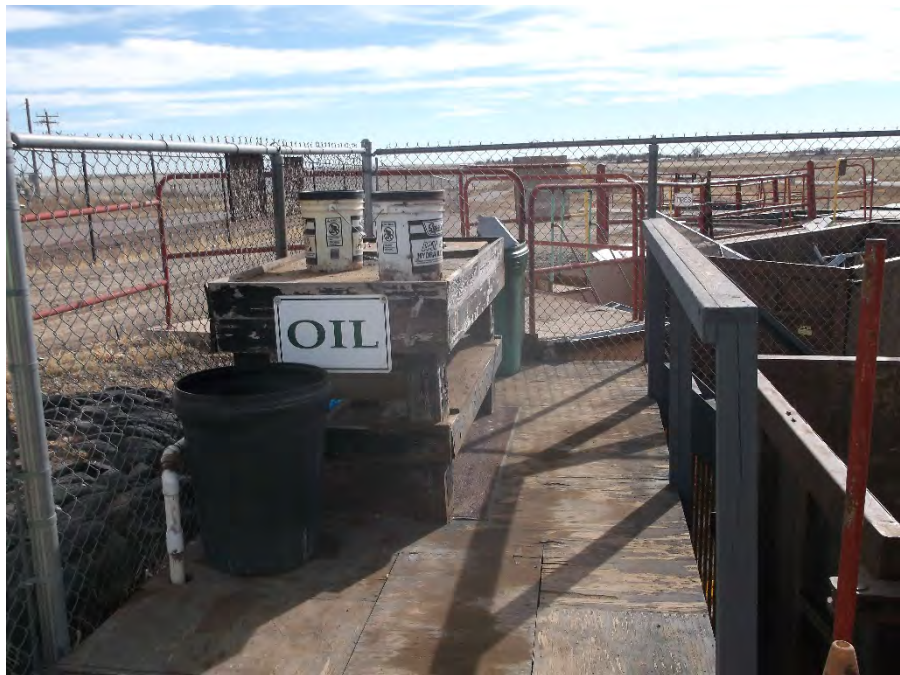
Oil Storage Facility
